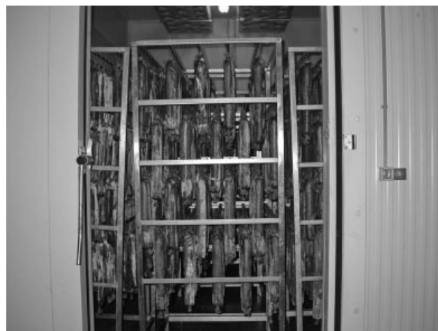
Figure 18.5. Example of a fermentation/drying chamber with computer control of temperature, relative humidity, and air rate. (By courtesy of Embutidos y Conservas Tabanera, Segovia, Spain.)
